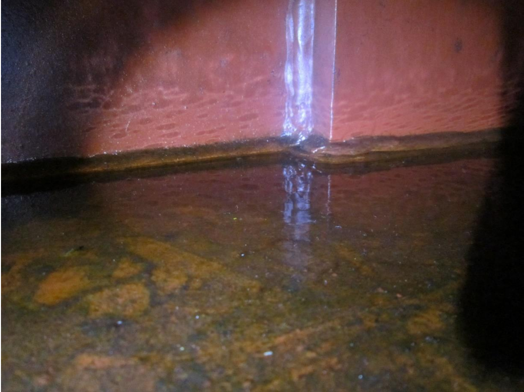
Figure 12. Oil Found on the Bottom of Unit 2 Generator Frame
