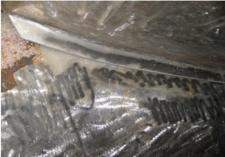
Figure 24. Additional Photo Showing Wicket Gates and Stay Vane with a Corrosion Patina
