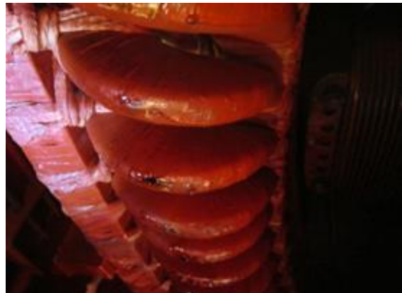
Figure 9. Unit 2 Lower End-Windings
