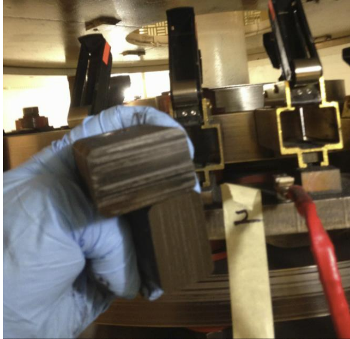
Figure H-1. Brush threading and uneven wear
