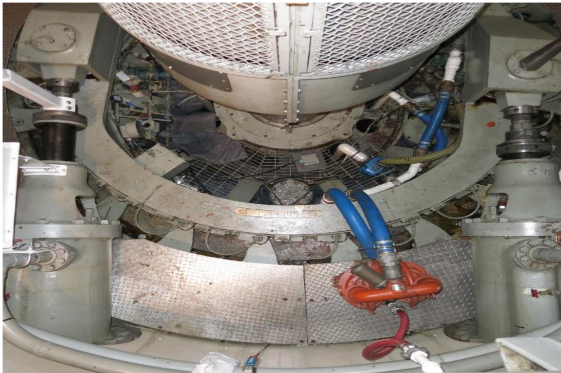
Figure 27. The Turbine Pit Showing the Two Wicket Gate Servos and the Wicket Gate Linkage.
