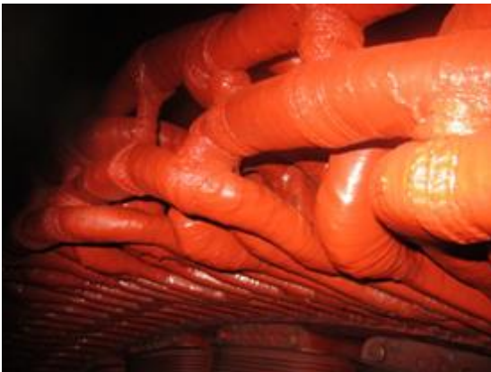
Figure 8. Unit 2 Upper End-Windings and Connection
