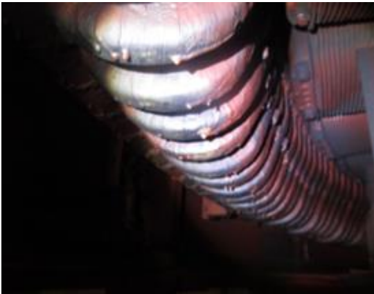
Figure 6. Unit 1 Lower End-Windings
