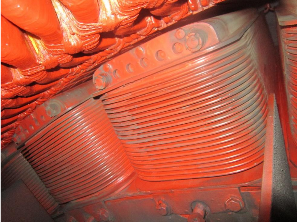
Figure 10. Unit 2 Rotor Poles
