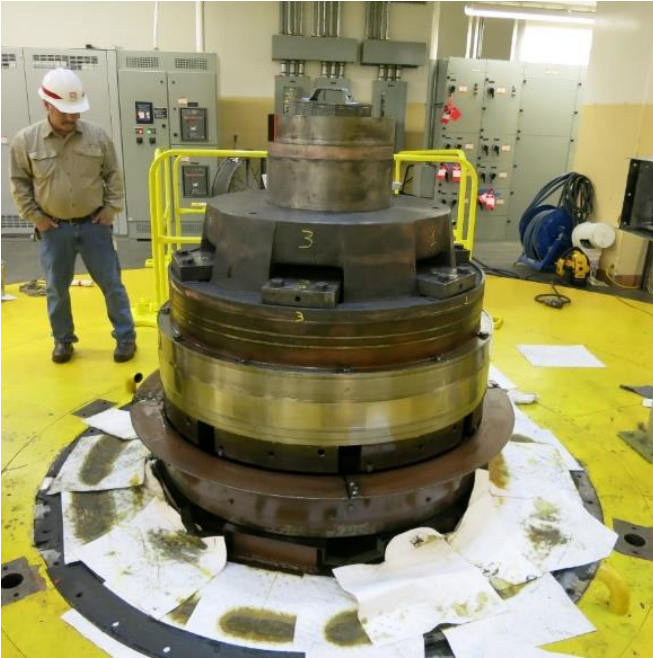
Figure 25. Unit 2 Disassembled Showing the Combination Generator Thrust Bearing/Upper Guide Bearing
