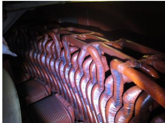
Figure 7. Unit 1 Upper End-Windings and Connection
