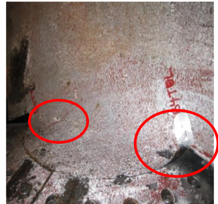
Figure 21. Blade Cracks That Have Been Repaired and Are Not Re-Cracking
