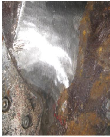
Figure 20. Paint Still Visible on the Runner Hub
