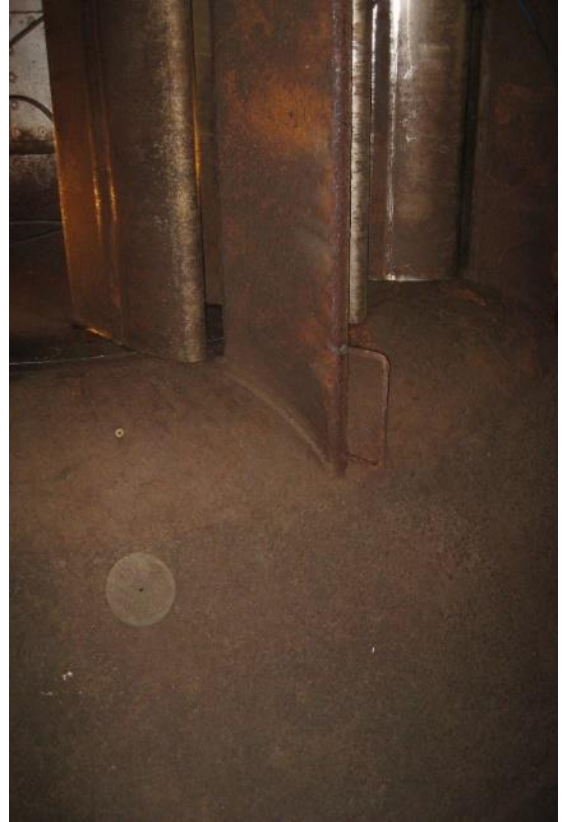
Figure 23. Discharge Ring SS Repair Shown Below a Blade with a Cavitation Fin
